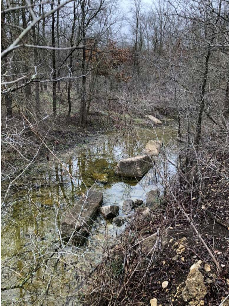
Figure 27. Site 41WM1435, disturbed concrete block remnants in Smith Branch Creek approximately 30 ft west of the railroad embankment, facing east/northeast. These remnants are believed to be from the bridge that carried the railroad over Smith Branch Creek, facing east/northeast.
