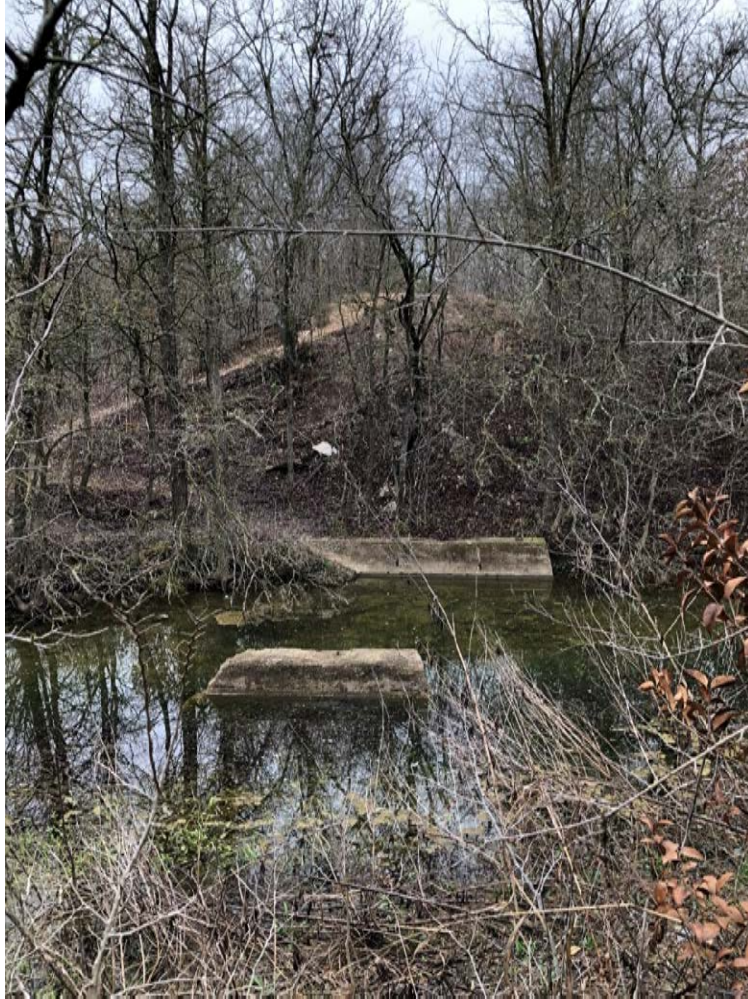
Figure 22. Site 41WM1435, remnants of the concrete railroad bridge substructure across Smith Branch Creek, facing north. Remains of the bridge are the concrete abutment and pier. Northern railroad embankment is evident beyond the creek at center with foot trail. Photo taken from top of railroad embankment at south bank of Smith Branch Creek.
