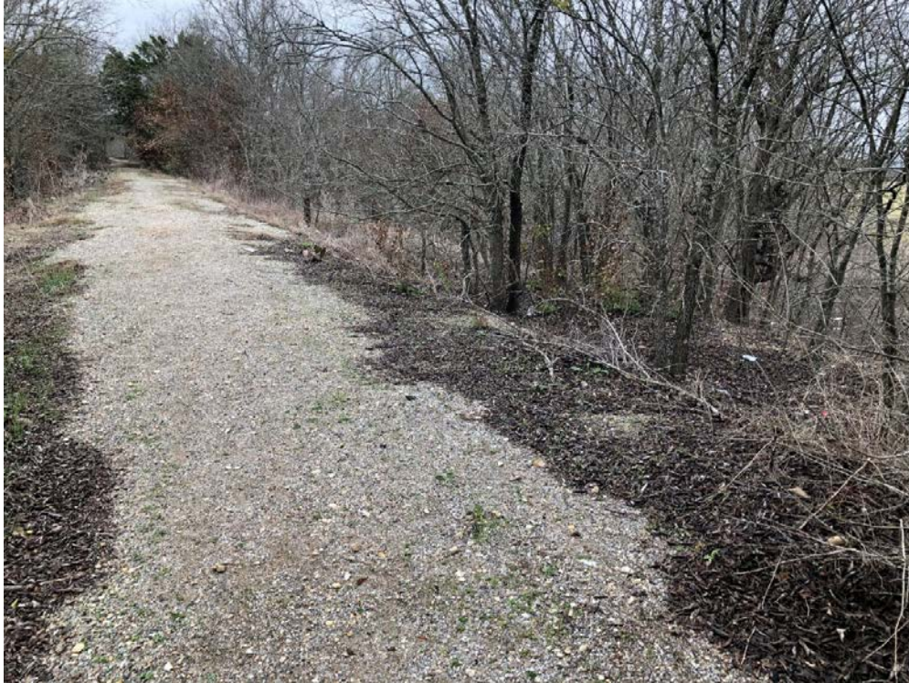
Figure 28. Site 41WM1435, railroad bed on top of the embankment approximately 250 ft north of Smith Branch Creek, facing south. Ballast is evident at surface.
